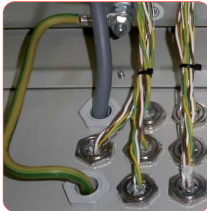
HF-Ground connection Control Panel Type "AE"
