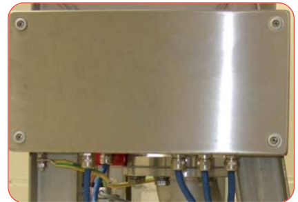
HF-Ground connection for Suppressor Junction-Box
