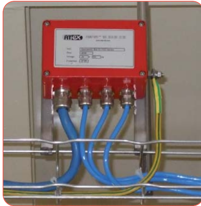
HF-Ground connection PXD Junction Box
